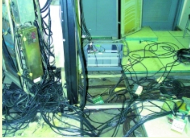
The weave of cables from cabinet to cabinet to power source were like a Gordian knot—almost impossible to untangle without a sword.
