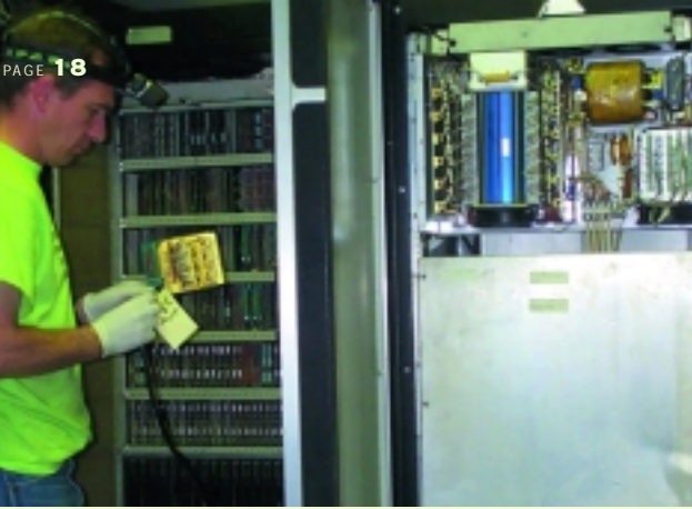
The cables were hard-wired into the cabinets and had circuit boards attached at various points.
